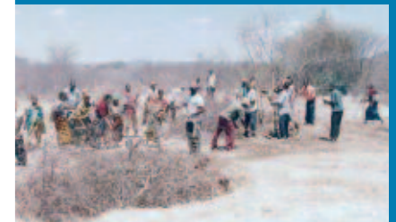
This is the site at Ovada village where the construction of the new dispensary has already started. Construction is also planned in Motto village (Sanzawa ADP) and Asanje (Mundemu ADP).
